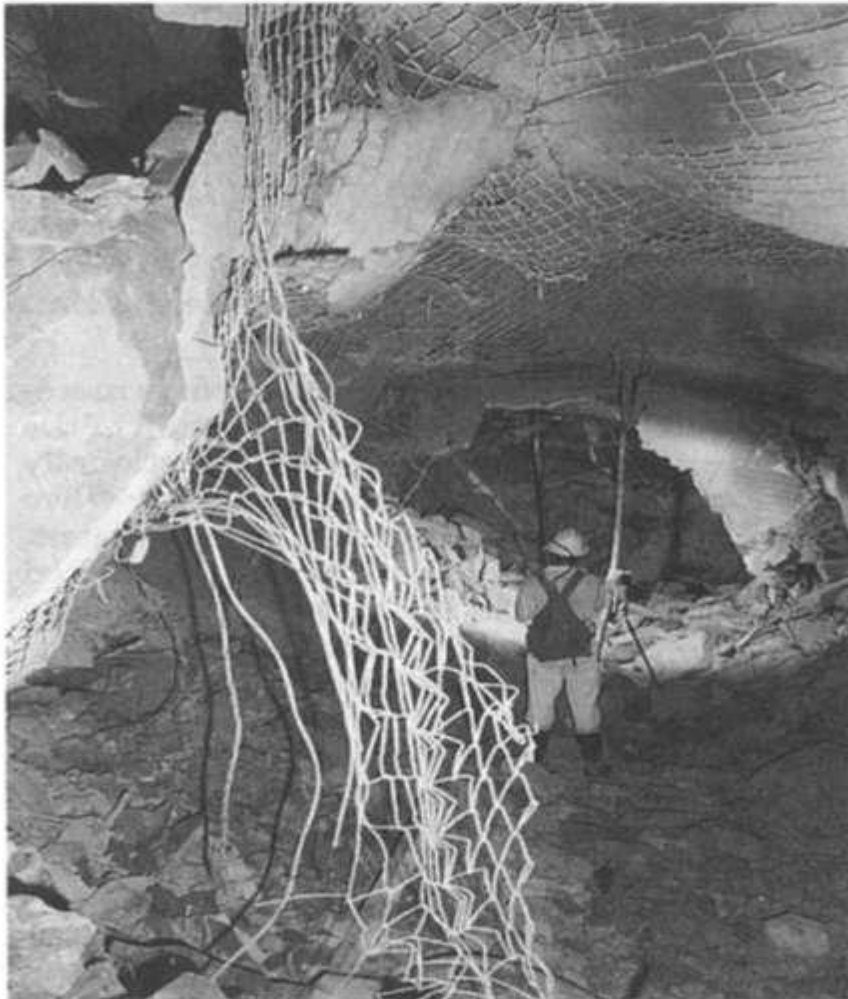
Fig: Face crush in 3.5 m x 3.5 m tunnel at a depth of 3100 m, after seismic event of 1.8 M L located about 40 m away.
